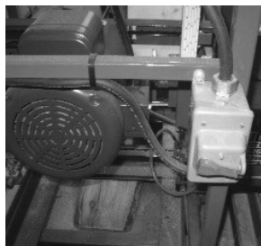
Electric mill, 220 volts, on/off switch.
